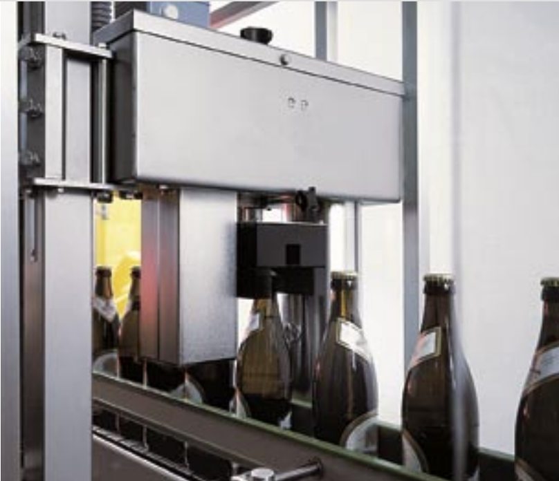
Measuring bridge for fill level inspection with the x-ray system, and closure inspection
